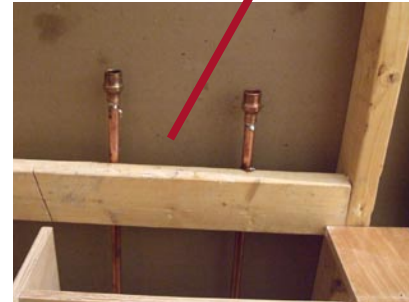
Note: hot and cold water supply lines have 3/4 " male (MIP) ends (on/off shut-off valves can also be installed here)
