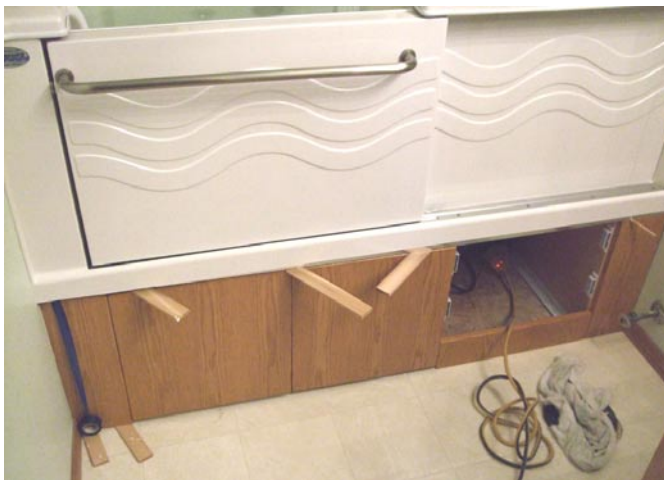
Tub and drain system on top of cabinet base and connected. Cabinet front panels being installed
